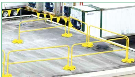
Temporary guard rail systems are often used to keep workers from going over the edge.
