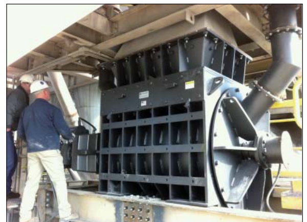
A PMCA-48 raw mill feeder at a cement plant.
