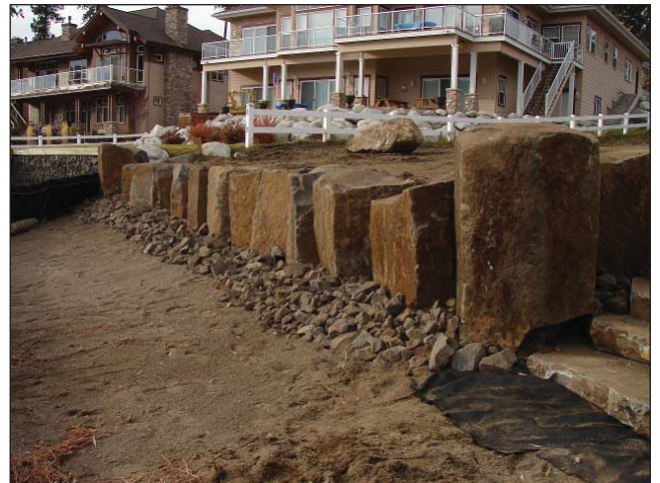
NIM can construct natural looking retaining walls to keep your property safe from wake water, waves and varying water levels.
