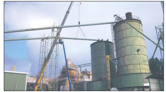
An employee is installing blow pipe to a flat back for the Silo.
