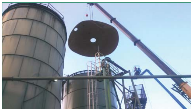
Putting the top on this silo is a tall job, but completed with competence and experience.
