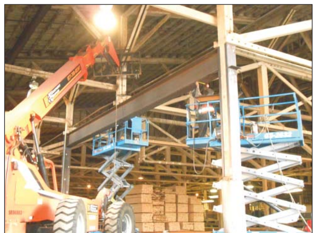
Mann Industrial replaced old wooden beams with structurally sound steel beams at Idaho Forest Group (IFG) in Lewiston, ID.
