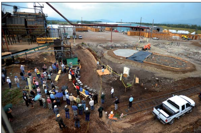
Overview of the ground breaking celebration of the Co-Generation Plant at F.H. Stoltze. The Co-Generation plant is expected to produce about 1% of the Flathead Electric Cooperative's total load.
